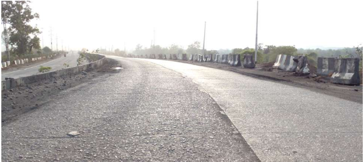
Concrete road of length 2700m and width 12m from Bankibahal towards Raigarh for HMV
